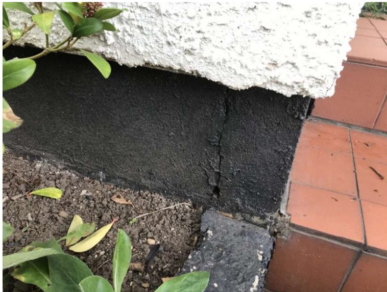
7.4. Crack to porch corner – thermal shrinkage
