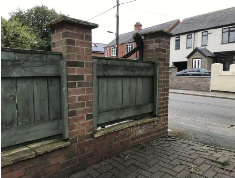
7.9. Crack and "broken back" to right boundary wall
