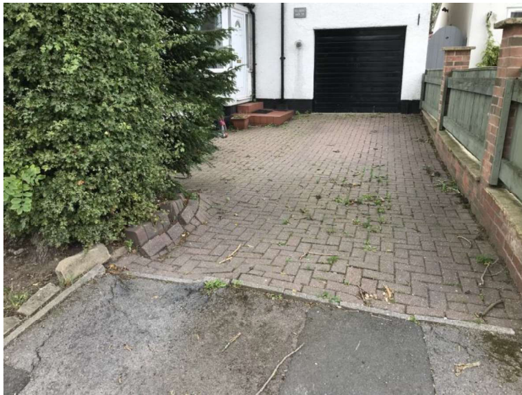
7.6. Damage to drive and highway pavement through tree root action
