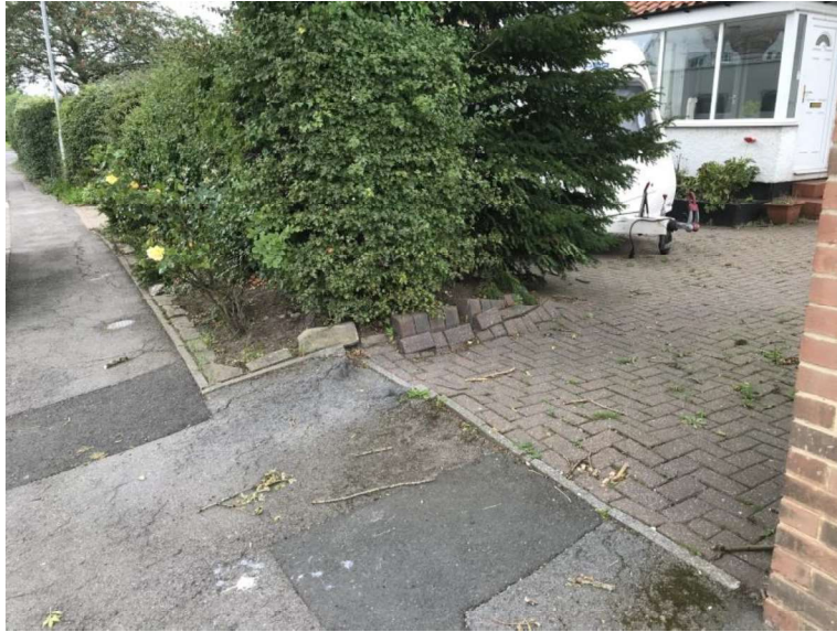
7.7. Damage to drive and highway pavement through tree root action
