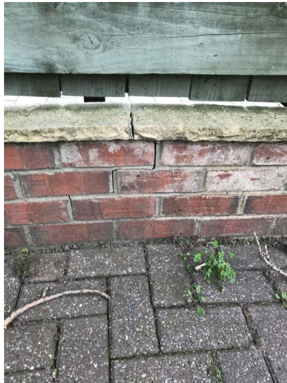
7.8. Crack and “broken back” to right boundary wall
